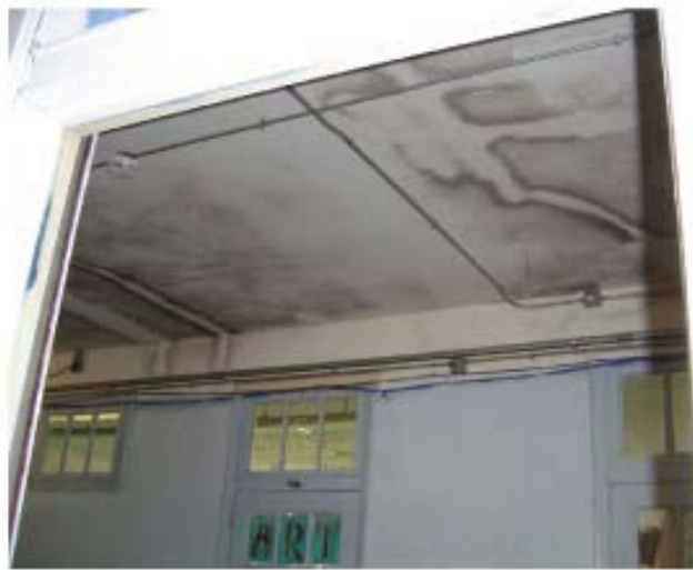
Figure 1. Picture of mold growing along fourth floor hallway ceiling at AFSHS
