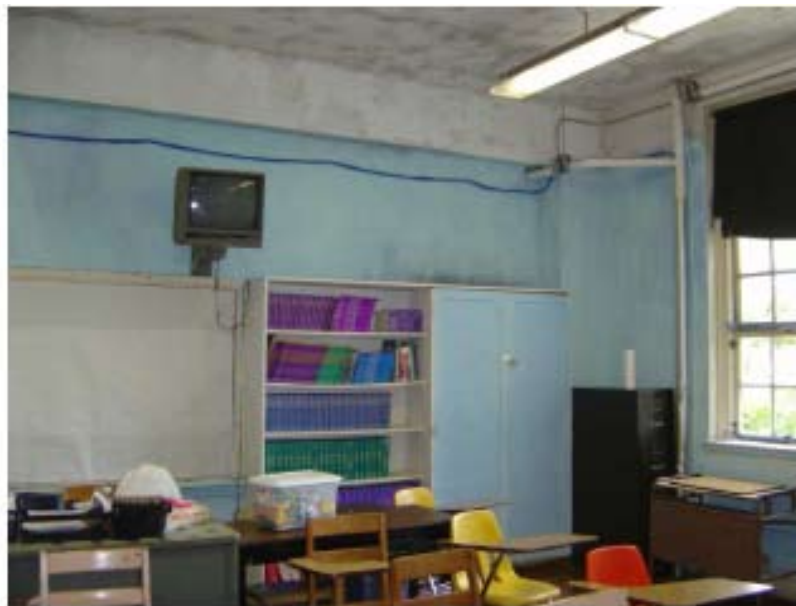
Figure 2. Picture of fourth floor classroom wall and ceiling showing active mold growth at AFSHS
